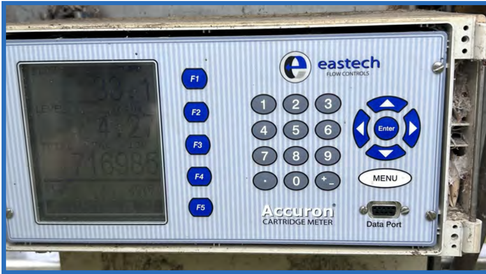
Leachate Collection Flow Meter Control Panel for Increment 1
