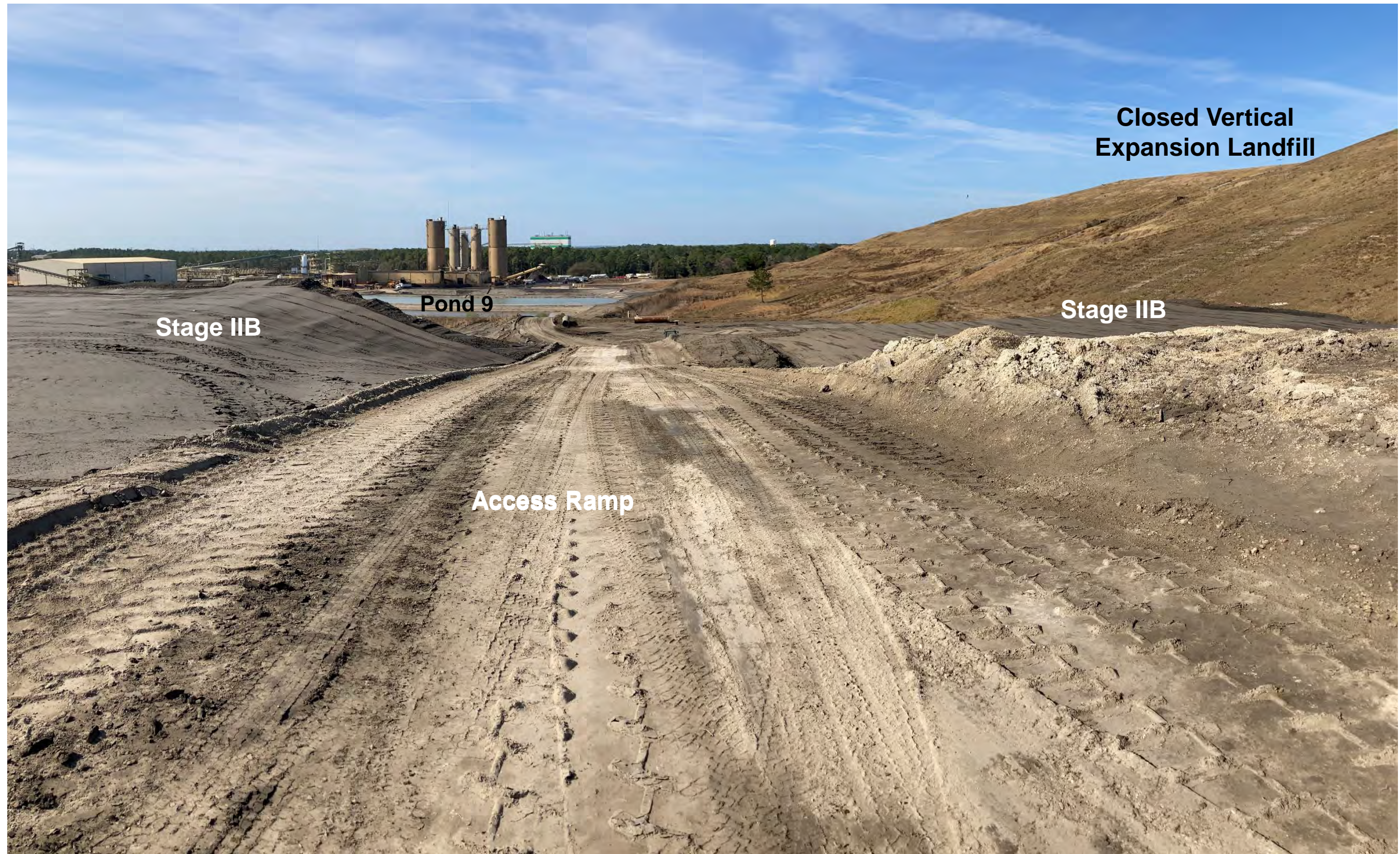
Access Ramp to Top of Stage I and Stage III, Looking Downhill to the West
