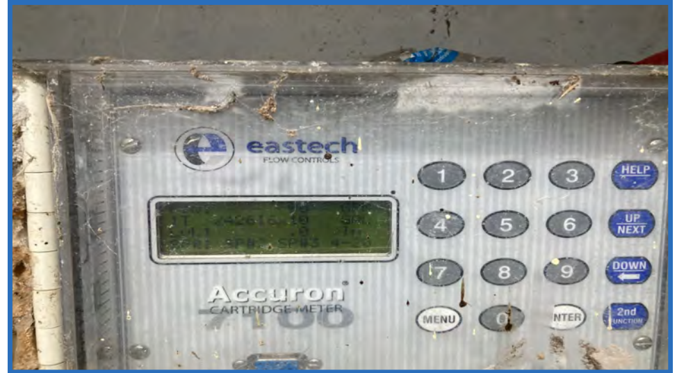
Leak Detection Flow Meter Control Panel for Increment 1
