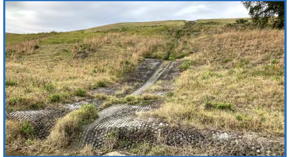
Fabriform-Lined Flume from Top of Closed Vertical Expansion to Stormwater Pond B, Looking Uphill from Perimeter Road
