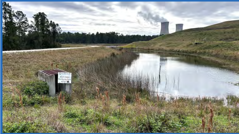
Outlet Structure CS-1 and Staff Gauge for Stormwater Pond B, Looking South
