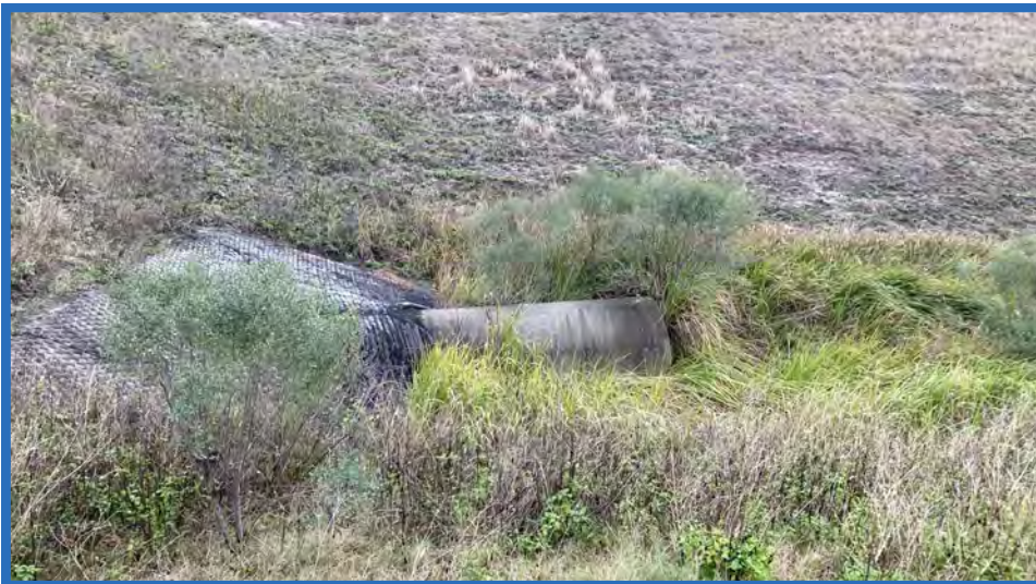
Fabricform Around Reinforced Concrete Pipe Under Access Ramp to Stage IIB, Looking East
