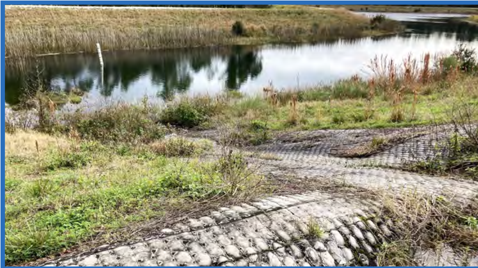
Staff Gauge for Stormwater Pond B and Fabriform-Lined Flume into Stormwater Pond B, Looking Southeast
