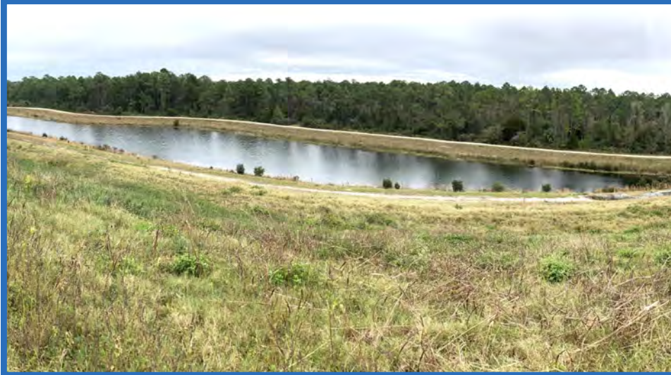
Side Slope of East Containment Dike for Stage I and Adjacent Perimeter Road, Looking Northeast from Bench Toward Stormwater Pond B
