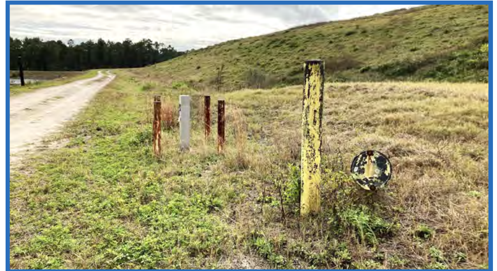
Monitor Well MW-22 and Leachate Collection System Cleanout East of Perimeter Road, Looking South with Stormwater Pond B to the Left
