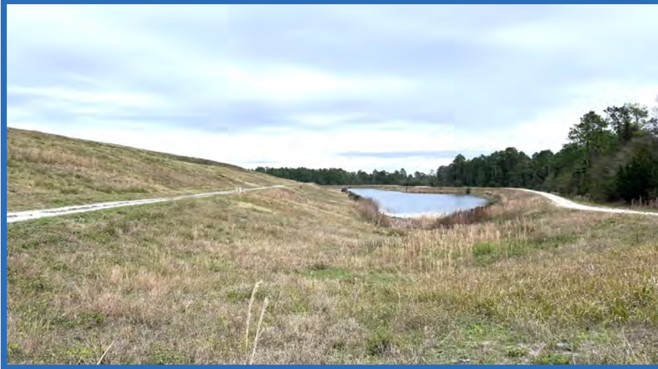
Perimeter Road, Eastern Slope of Containment Dike for Stage I, and Stormwater Pond B, Looking North
