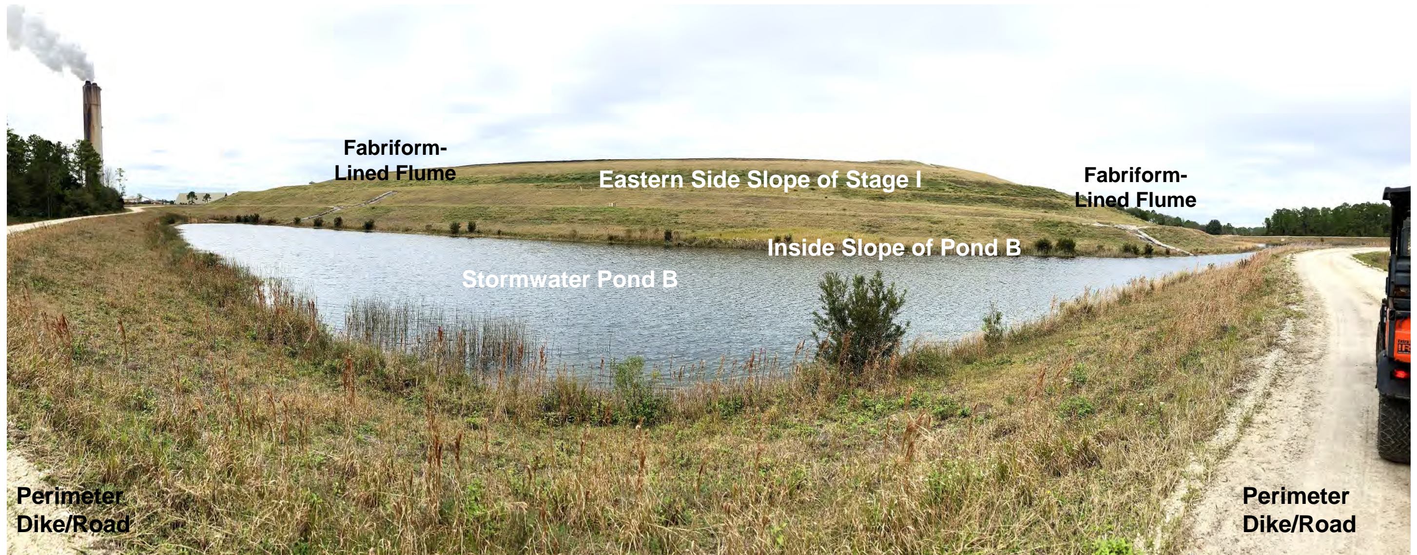
Increment 1, Stage I Eastern Side Slope and Containment Dike, Looking West from Perimeter Dike/Road on the Other Side of Stormwater Pond B
