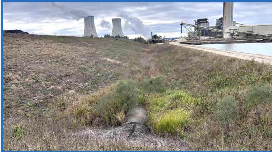
Containment Dike for Stage IIB, Perimeter Swale, Perimeter Road, and Culvert Looking South
