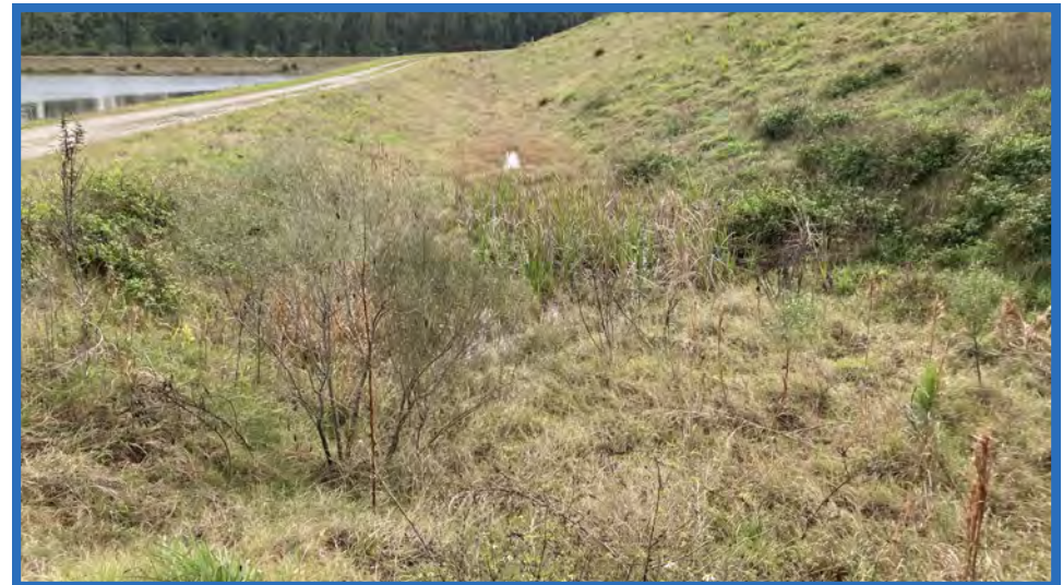
Sump Area of Increment I and Perimeter Swale East of Stage I, Looking Southwest
