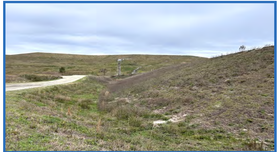
Perimeter Swale Along Toe of Western Containment Dike for Stage IIB, Looking North Toward Closed Original Landfill and Vertical Expansion
