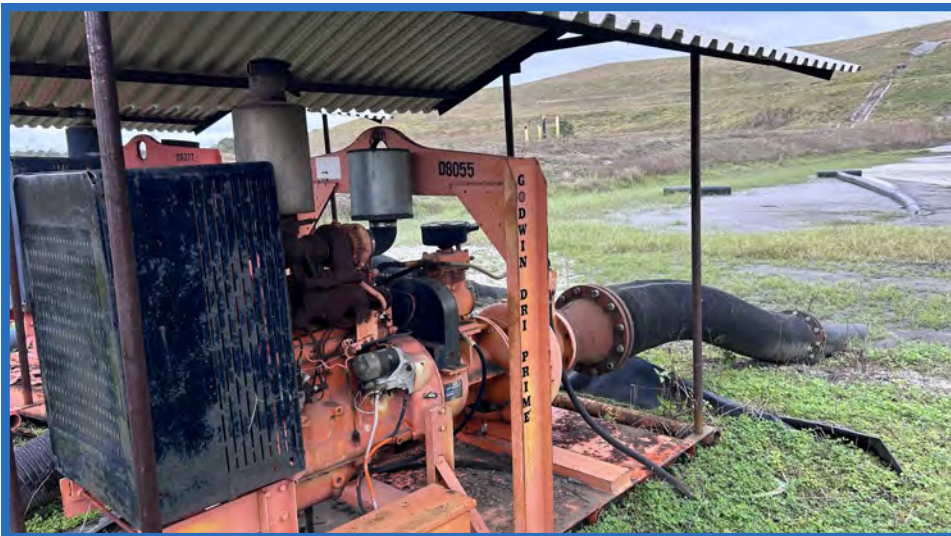
Auxiliary Pumps with Intake Pipelines in Low Point of Stage IIB
