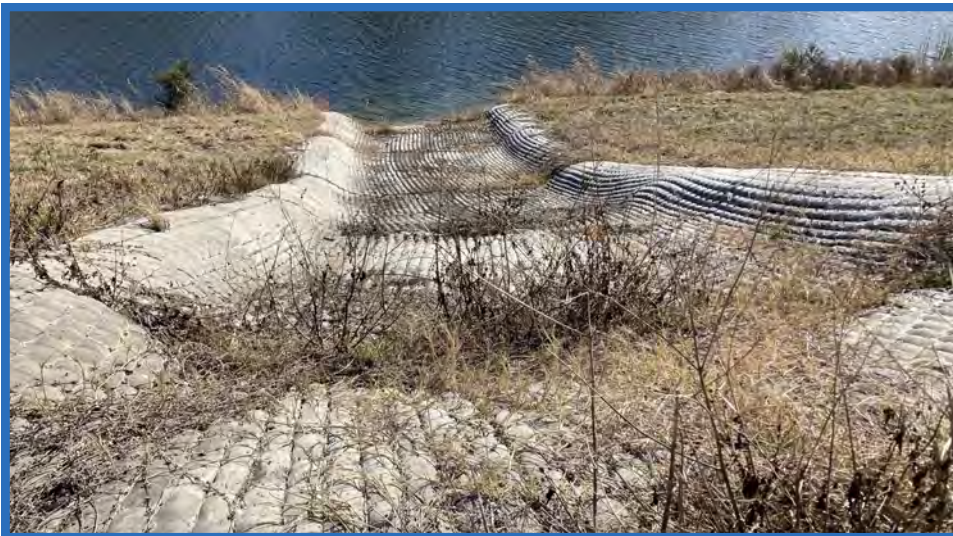
Fabriform-Lined Flume from Southern Part of Eastern Containment Dike of Stage I into Stormwater Pond B, Looking East
