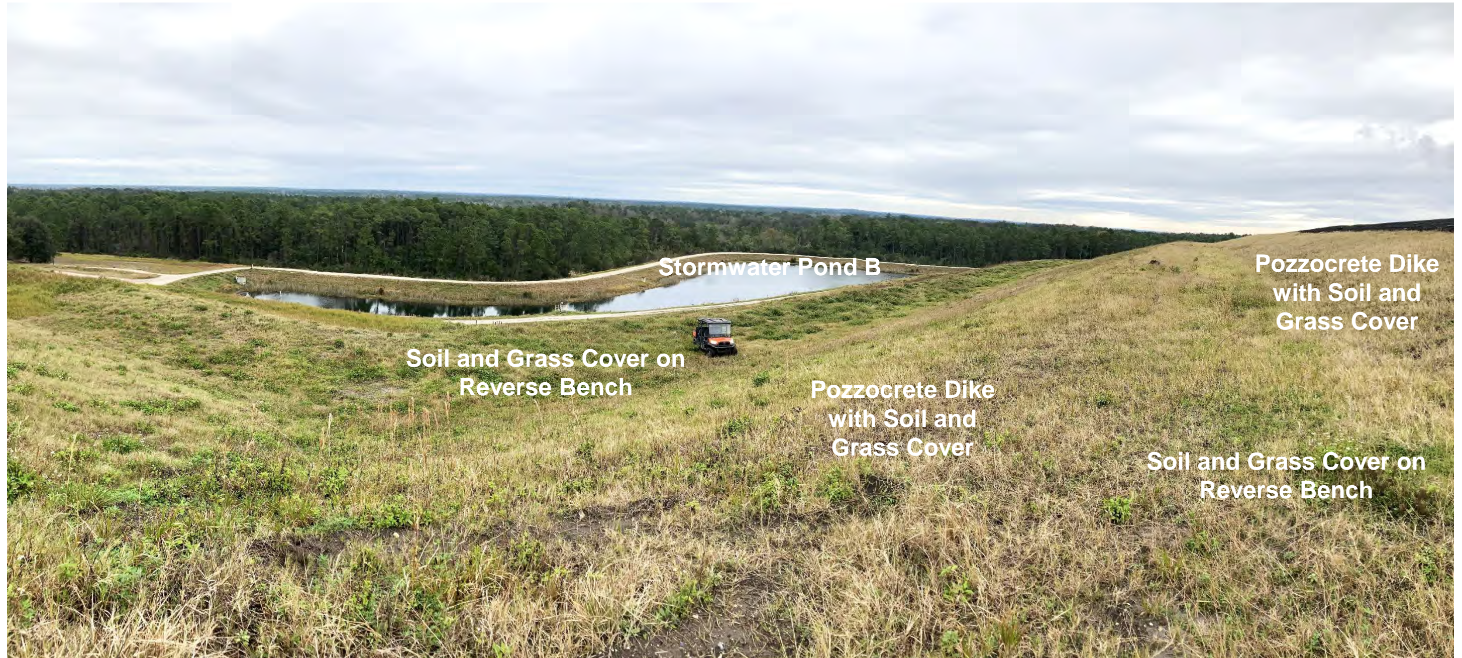
Pozzocrete Dikes and Reverse Benches on East Side of Increment 1, Stage I, Looking Southeast Toward Stormwater Pond B
