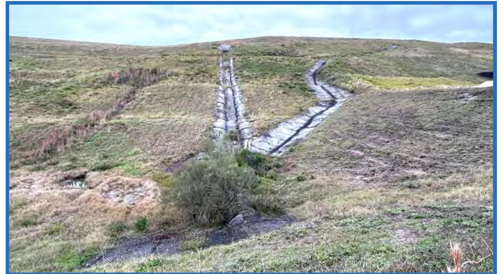
North End of Western Containment Dike for Stage IIB and Fabricform-Lined Flumes, Looking North
