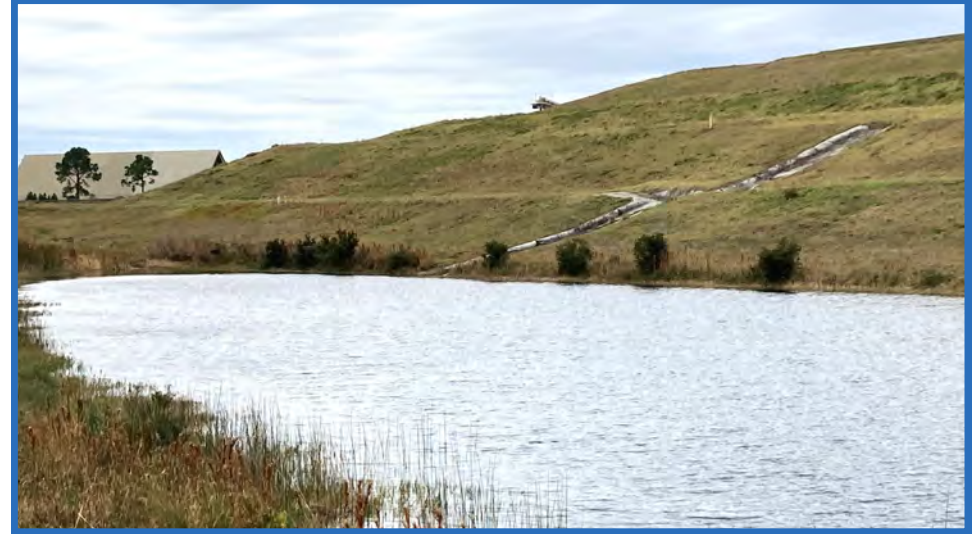
Eastern Slope of Increment 1 and Fabriform-Lined Flume into Stormwater Pond B, Looking Southwest from Perimeter Road Around Eastern Side of Pond B
