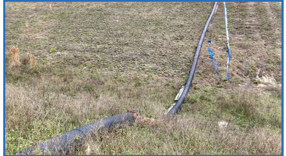
Pipeline from Auxiliary Pumps for Low Point of Stage IIB to Pond 9, Looking East
