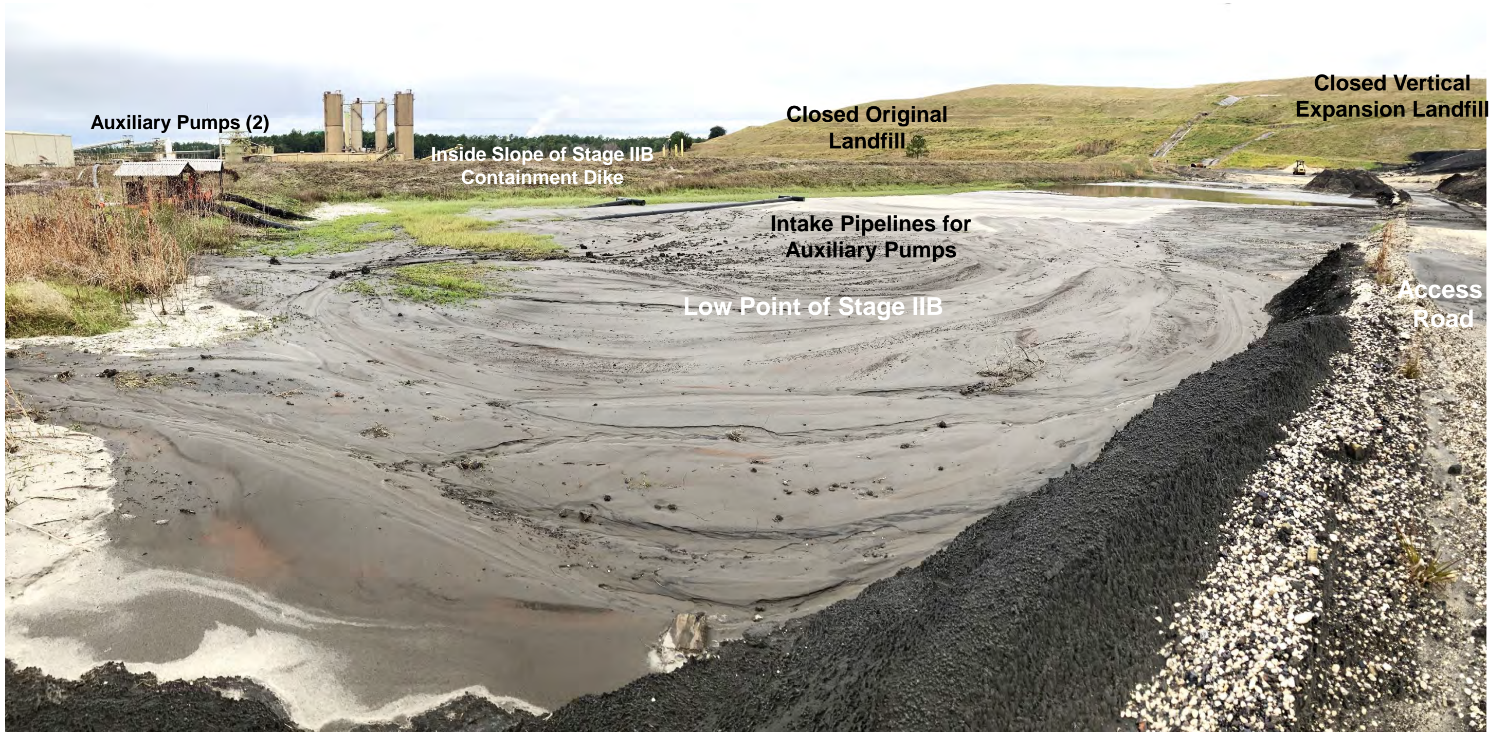
Pump Intake Pipelines in Low Point of Stage IIB, Looking West
