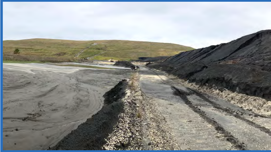
Access Ramp through Stage IIB and Western Extent of Waste, Looking North Toward Closed Vertical Expansion
