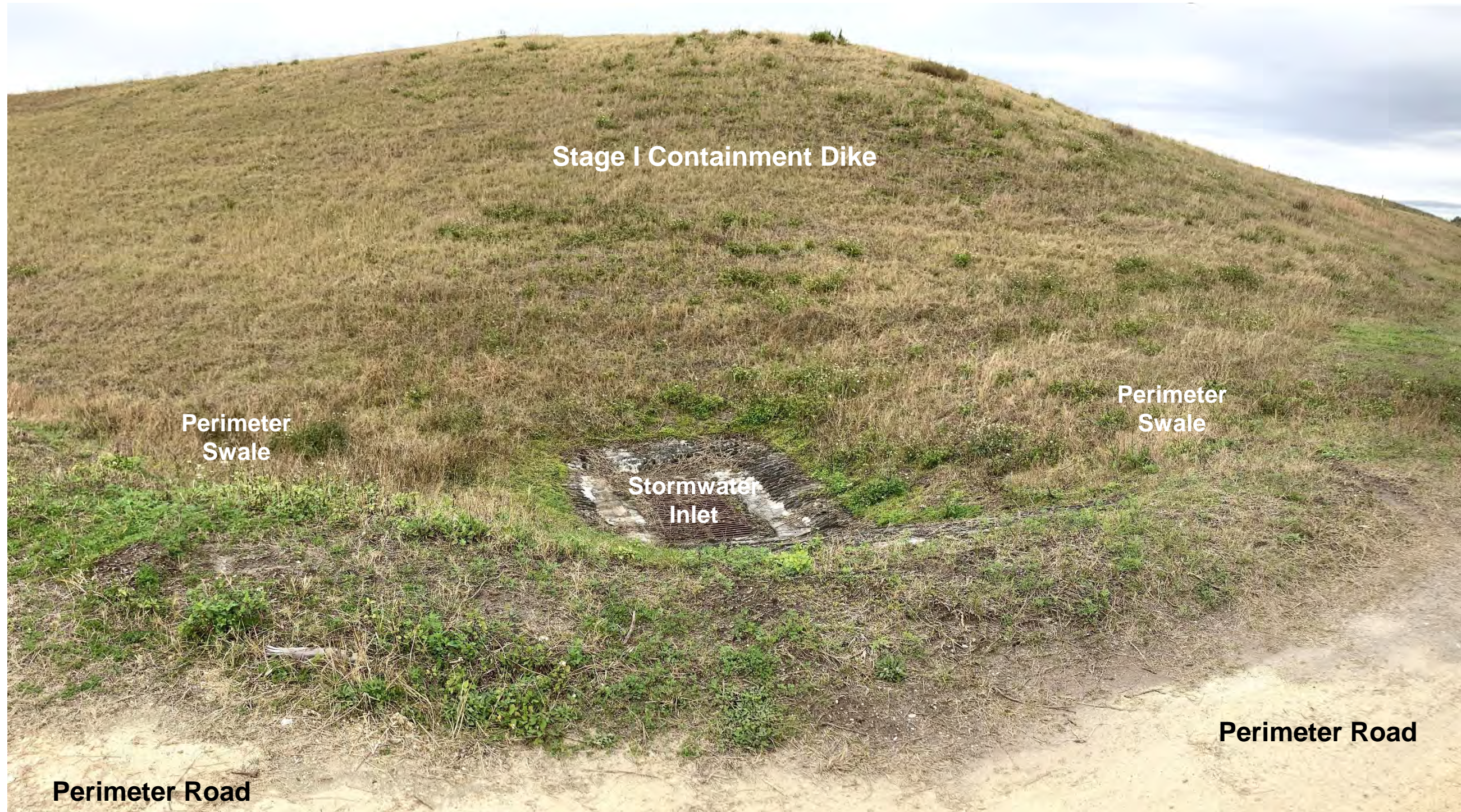
Stormwater Inlet in Perimeter Swale at Southeastern Corner of Stage I Containment Dike, Looking Northwest
