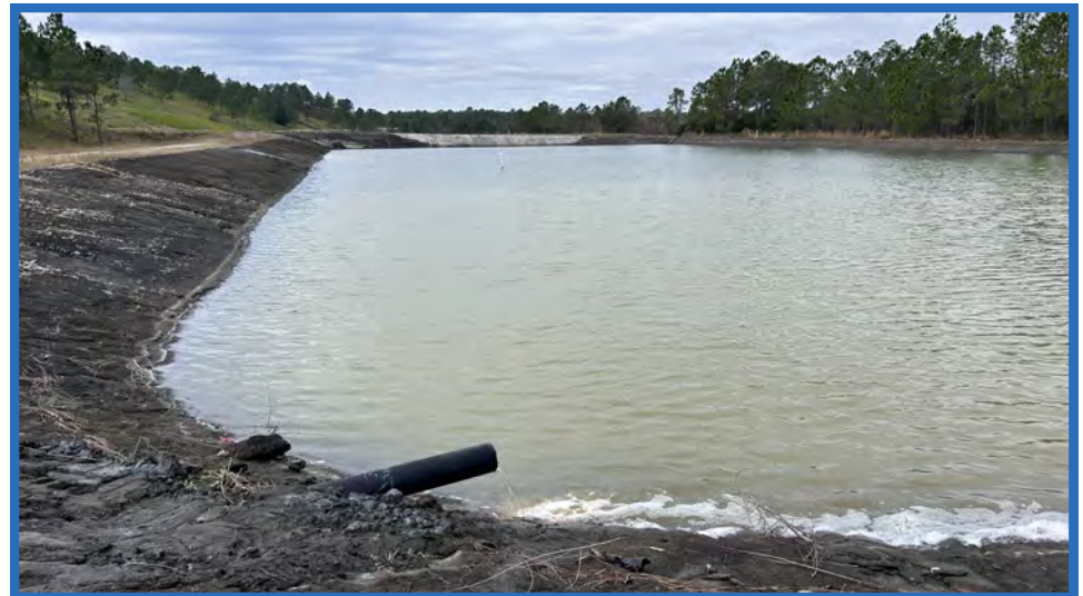
8-Inch Diameter HDPE Discharge Pipe from Increment 1 Leachate Collection and Leak Detection System into Pond 8
