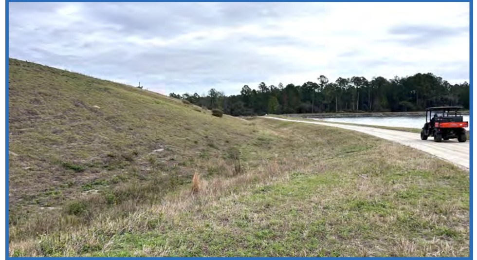
Perimeter Swale and Road at Southwestern Corner of Stage IIB Containment Dike, Looking Southeast
