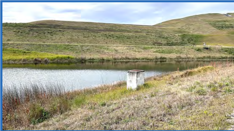
Outlet Structure CS-2 for Stormwater Pond B, Looking West from Perimeter Road Around Eastern Side of Pond B
